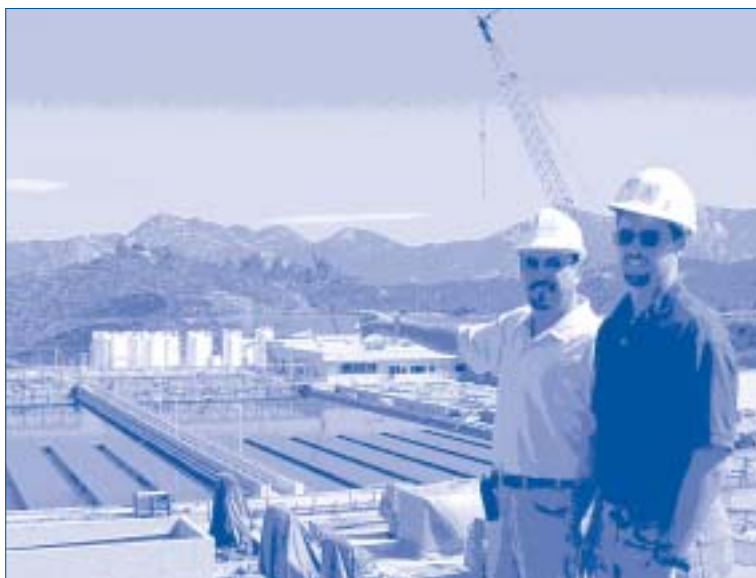
Moreno-Lakeside Pipeline Project Engineer Karem Elhams points out recent improvements at the R.M. Levy Water Treatment plant to Project Manager Gary Bousquet. Once completed, the improvements will enable the plant to treat additional water delivered by the future pipeline.
