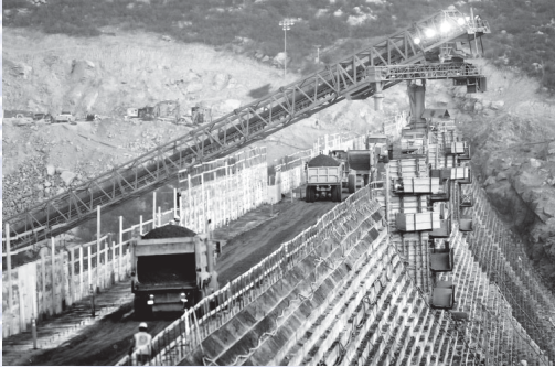
The dam raise will be constructed of roller-compacted concrete, which was also used on the recently completed Olivenhain Dam.
