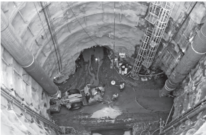
The Slaughterhouse Shaft (seen here) and the Central Shaft have been excavated to the depth of the tunnel, and the San Vicente Portal development is about 75 percent complete. Work on the West Shaft recently began.
