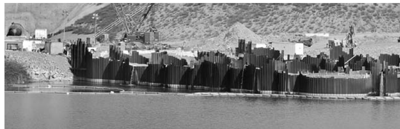
The temporary cofferdam holds back water while the inlet-outlet structure is built.
