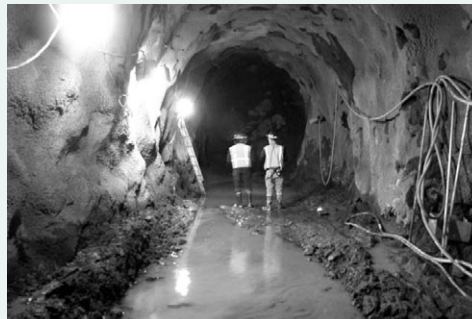
Tunneling is under way at four locations along the 11-mile pipeline route.
