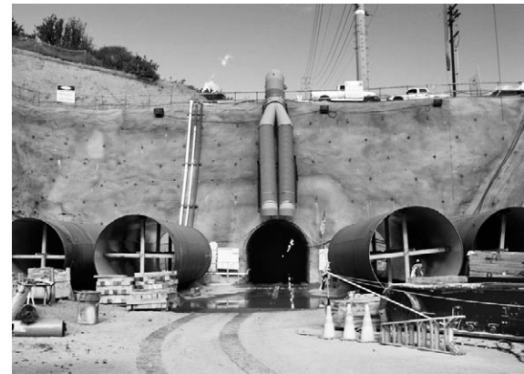
Pipe sections 10 feet in diameter are inserted one by one in the tunnel and welded together.
