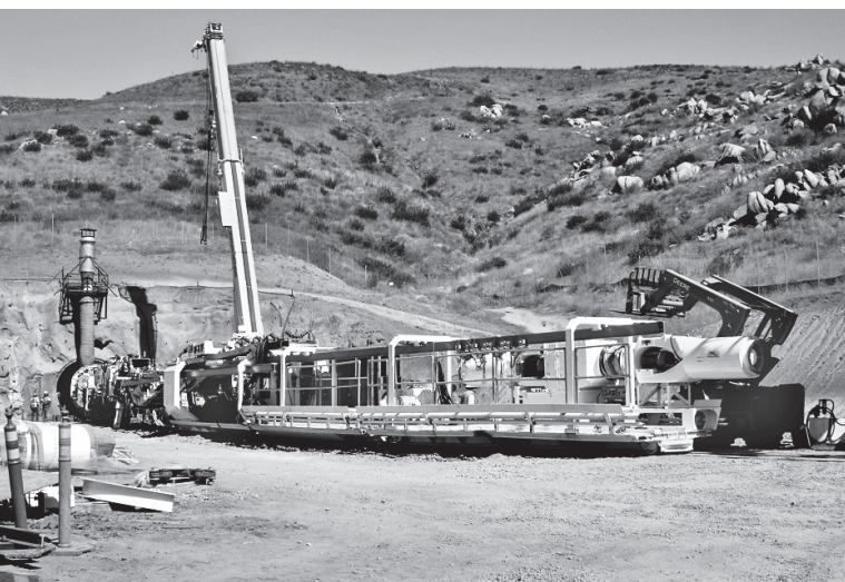
The tunnel boring machines have a long conveyor belt system to remove the dirt and rock from the tunnel.
