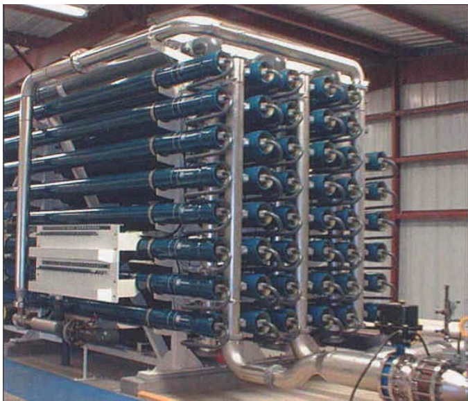
Demineralization of brackish groundwater in Oceanside.
