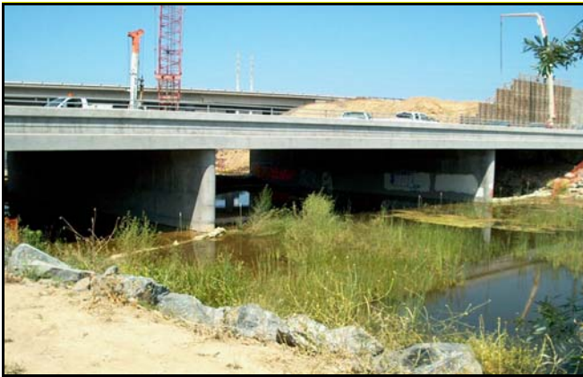
Figure 3-2. Los Peñasquitos Creek Mass Loading Station.
