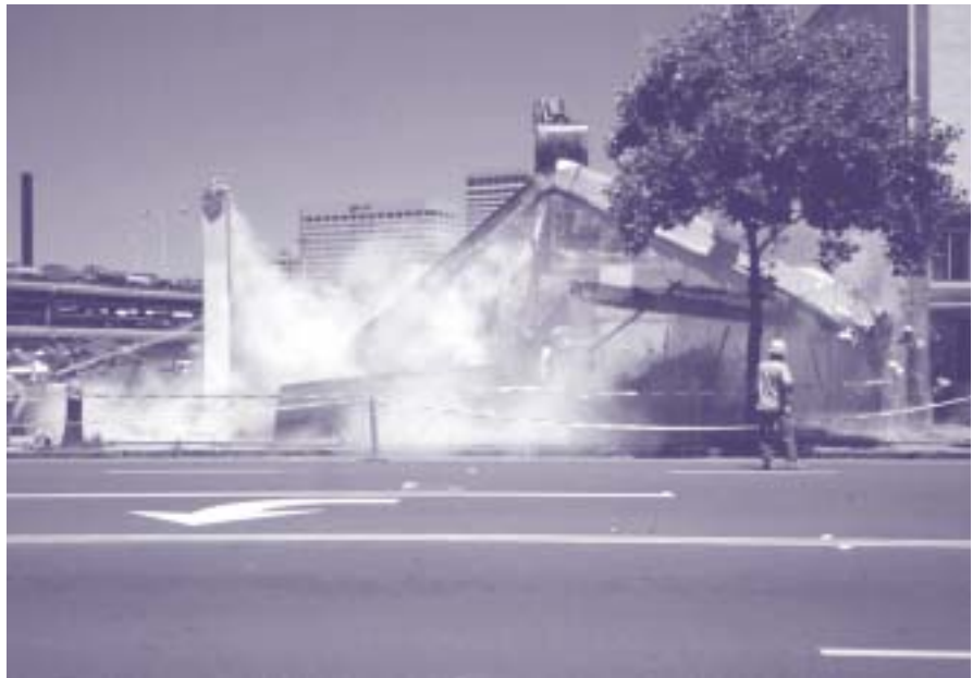
Several shops in Oakland, CA are demolished creating dust from brick, stucco, and plaster, all of which contain silica.
