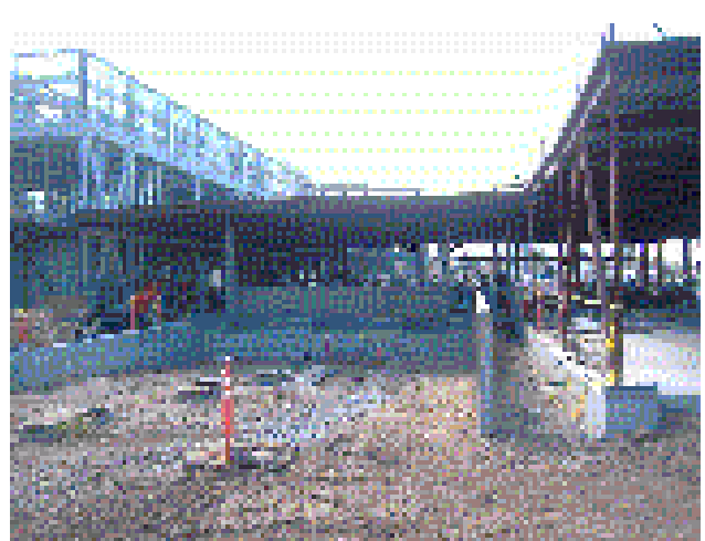
The loading dock is taking shape. Every truck coming to the facility will make their deliveries here.
