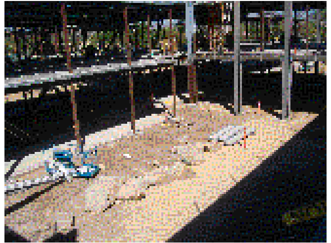
The facility is built around four interior courtyards. This is a view of one of the interior courtyards from the second floor.
