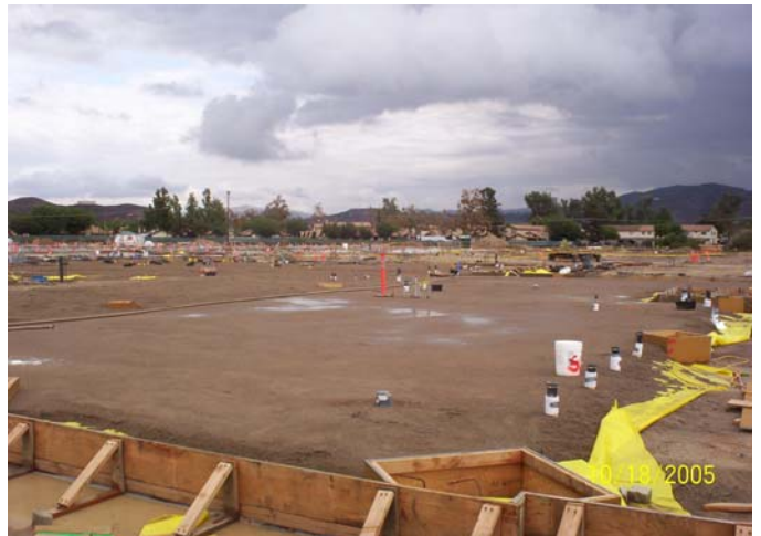
Puddles on the Slab of Building Three
