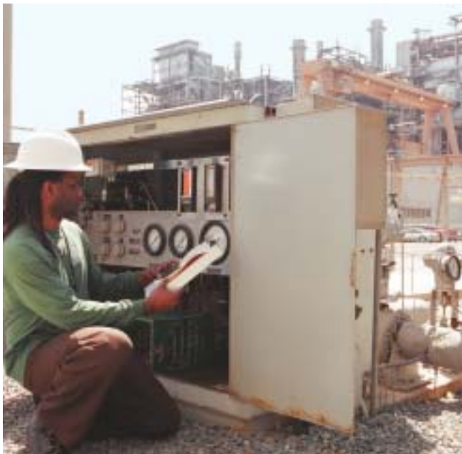
An air pollution engineer checks equipment at the South Bay Power Plant. Power generation contributes to air pollution.
